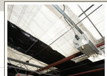
The use of blackout curtains on this greenhouse helps to reduce the offsite impact of grow lights.
