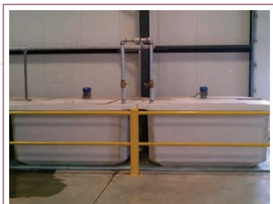
Locate stock tanks in areas with minimal or no traffic, and protect them from accidental impact.
