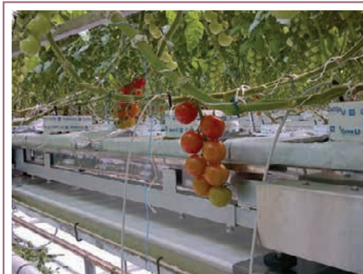
For best results, use and monitor devices such as weigh scales that detect when fertigation should start.
