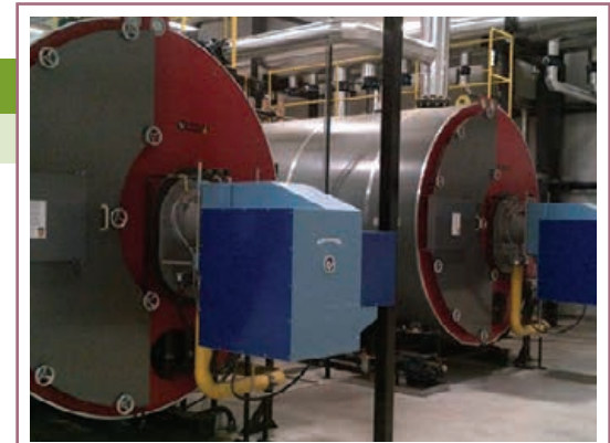
Regular boiler maintenance enhances heating efficiency.
