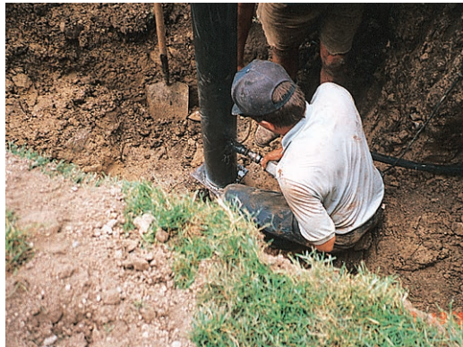
Consult a licensed water well contractor for advice and assistance with the extension of the water well casing.
