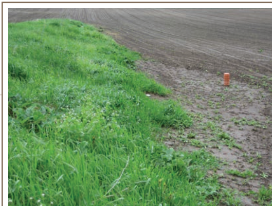
Surface inlets move excess surface water on cropland to subsurface drainage systems in a controlled manner that reduces soil loss.
