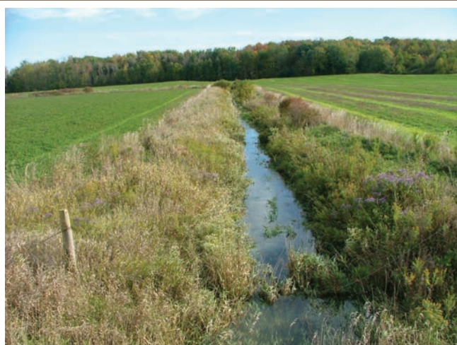
A thick cover of vegetation will stabilize the banks and greatly reduce maintenance requirements.
