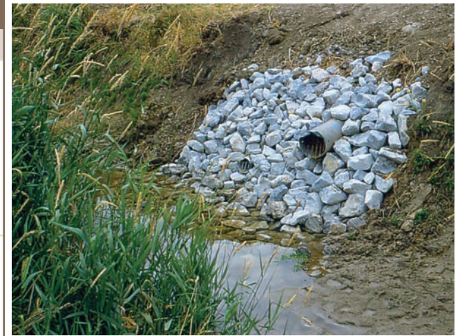
Proper placement and design of drainage outlets is important to prevent bank erosion and maintain stability of the outlet.
