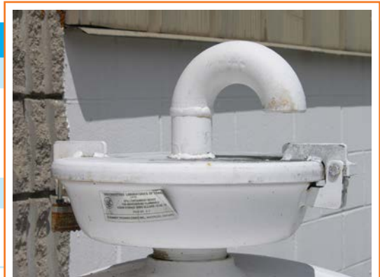
The overfill device is designed to prevent filling to more than 95% capacity.
