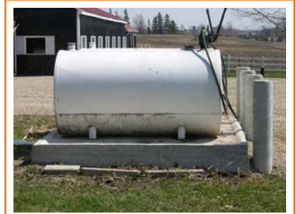
Locate fuel storage so it does not create a fire hazard for buildings.
