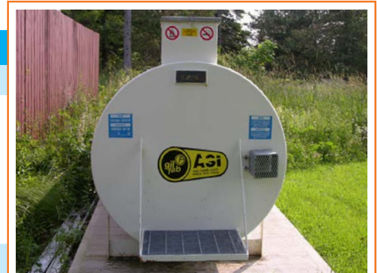
Evaluate condition of existing fuel storage tanks and maintain the corrosion protection.
