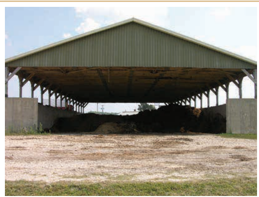
Eliminating direct rain and snowfall will free up available manure storage capacity.
