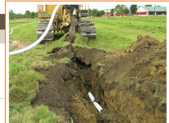
To reduce the risk of contaminants flowing into the tile and reaching surface water, maintain an adequate separation distance – greater than 15 m (49 ft) – between the disposal vessel and field drainage tile.
